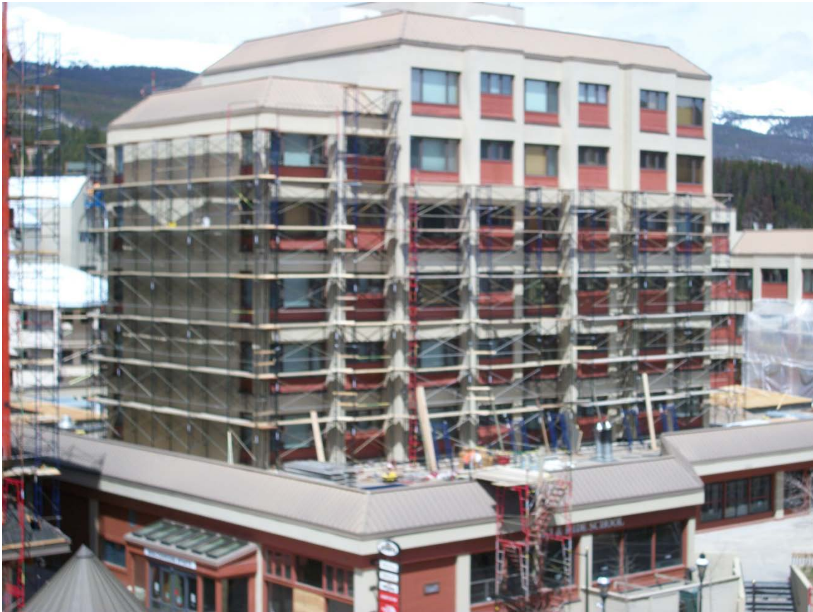
View of the East & South sides of Liftside as taken from the 5 th floor of scaffold on Plaza 1.
