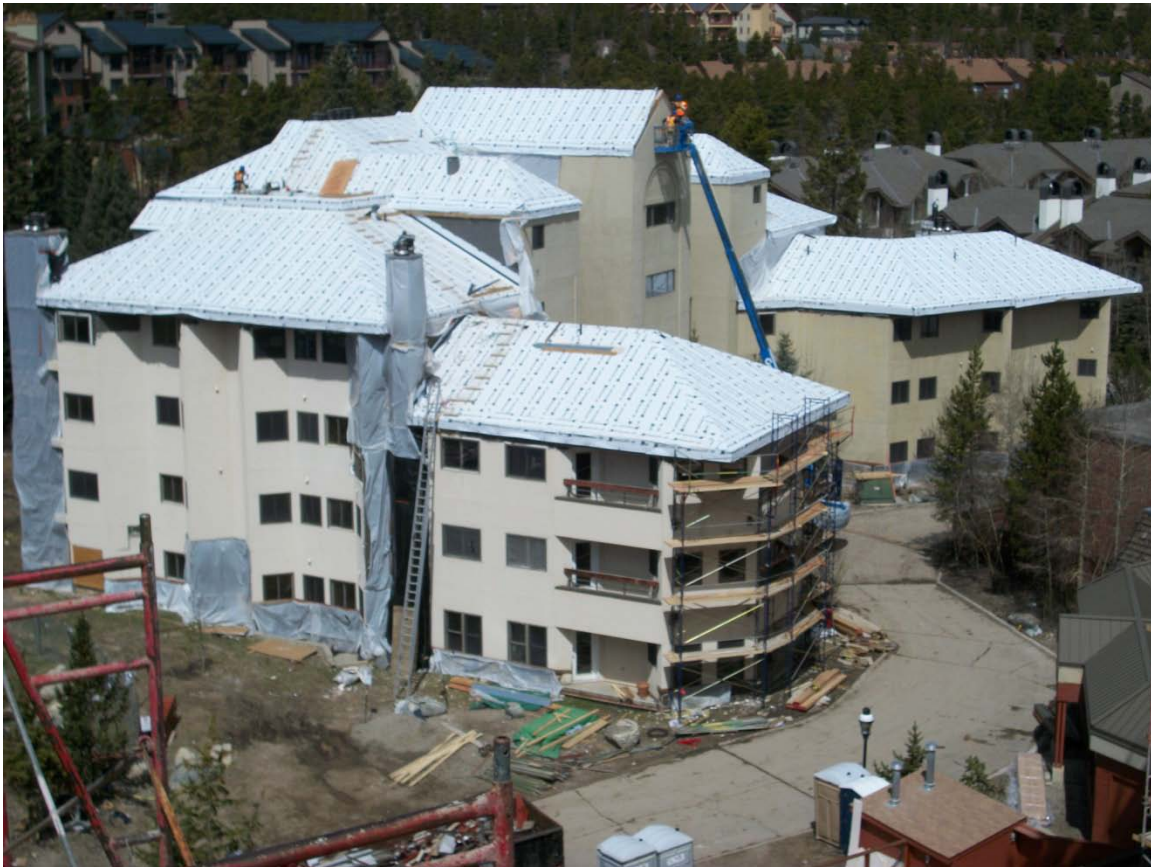
View of Chateaux taken from atop Plaza 2 roof. The entire roof and all adjacent walls have been dried in. Scaffolding has begun on the East (Entry) side of the building.
